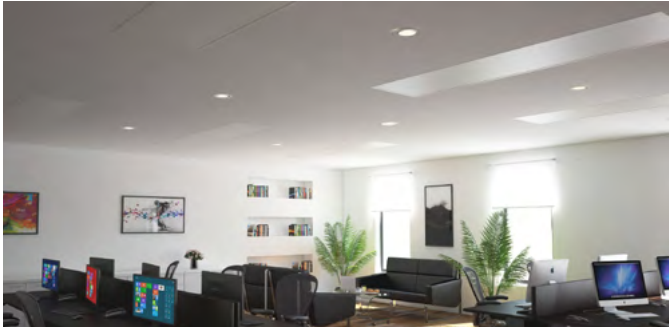
EFW Panels Recessed into Plasterboard Ceiling
